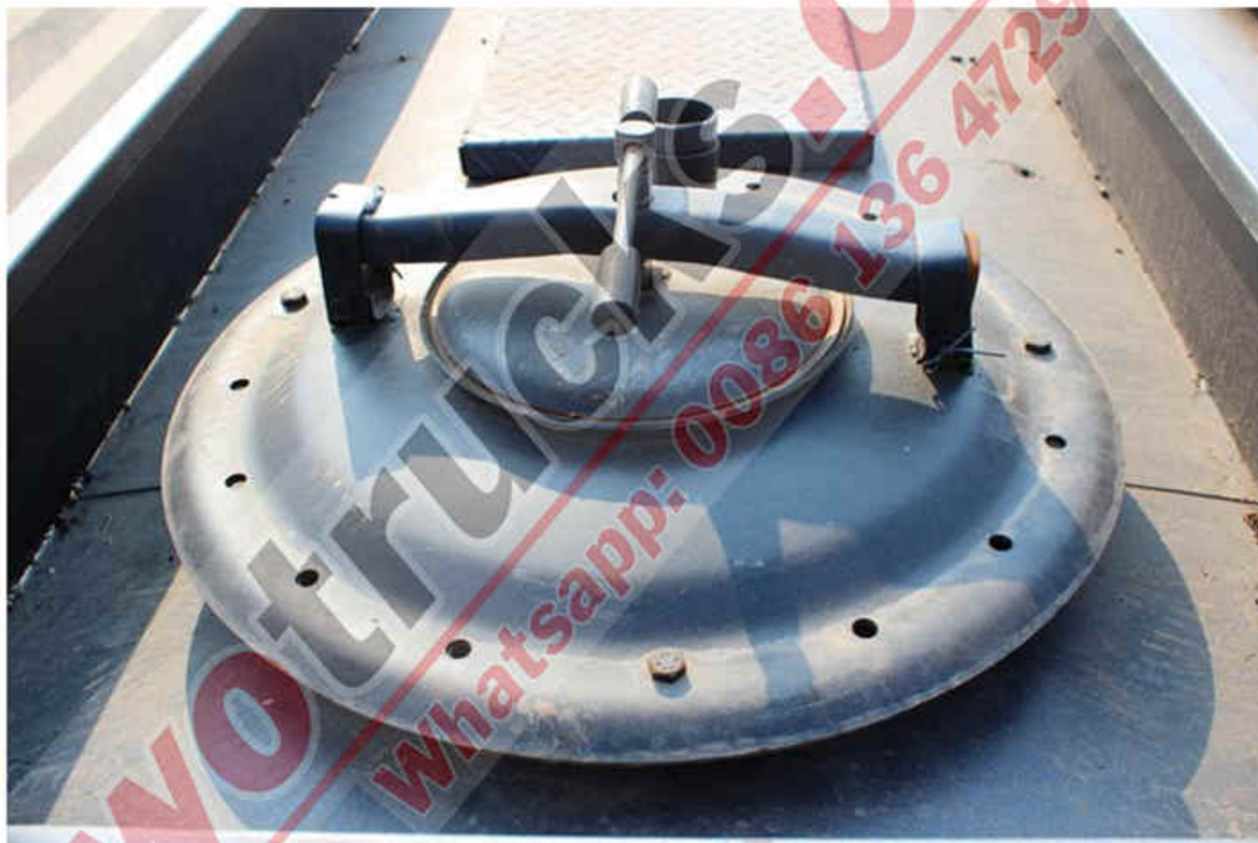
Fig. 7 Asphalt tank oil filler
