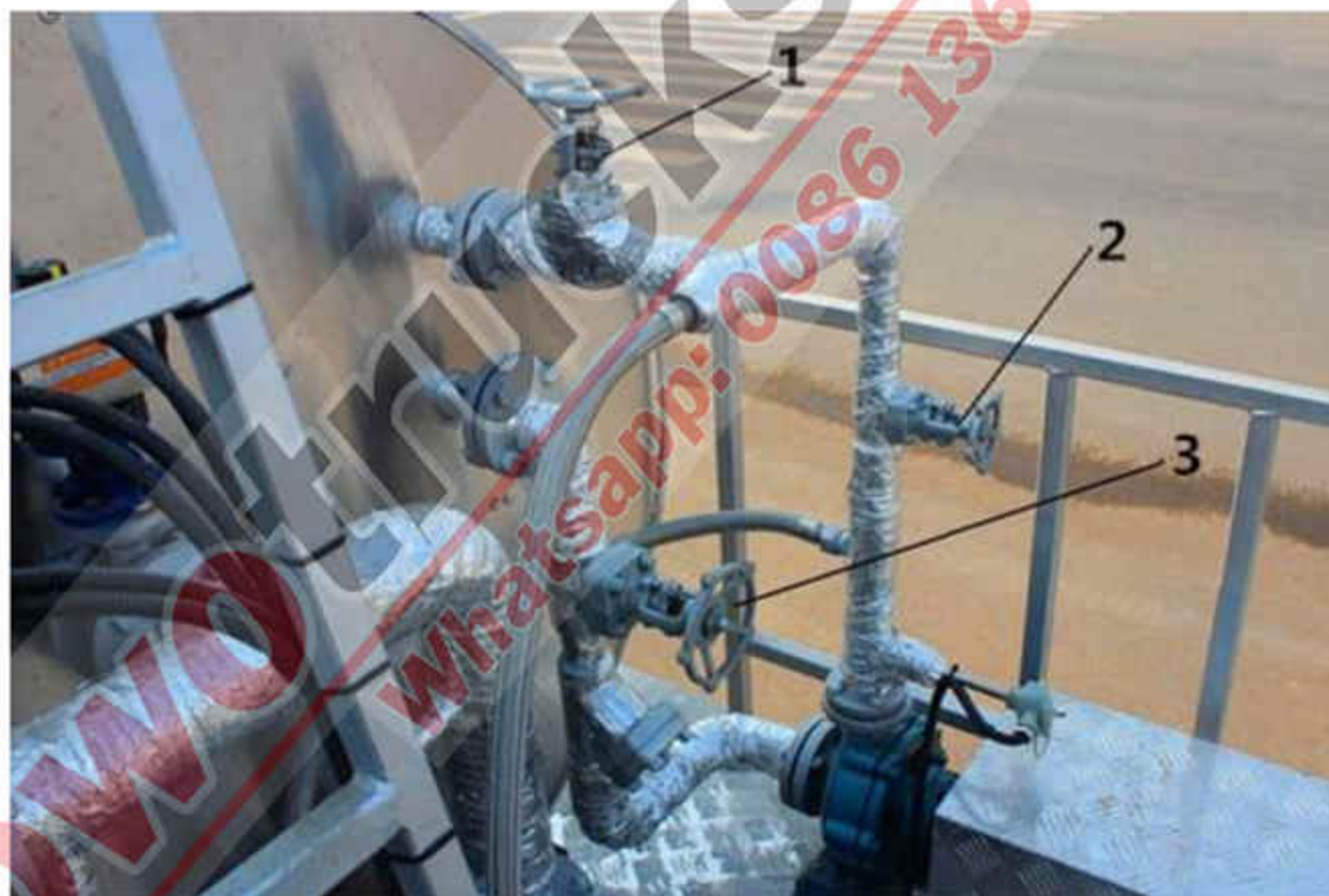
Fig. 11 Heat transfer oil valve
